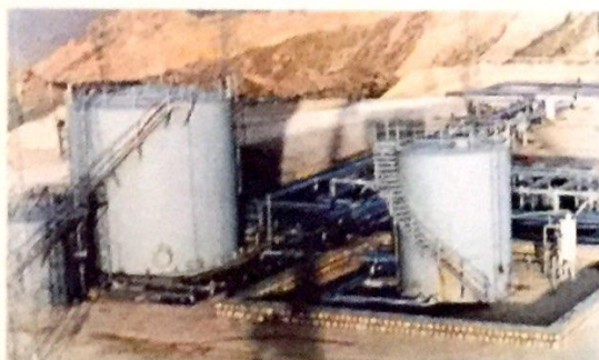
Figure 18: Gas Separation Unit at Kangan (Courtesy of Tehran Jonoub)
