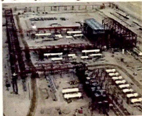
Figure 6 : Sarkhun 2 Natural Gas Refinery (courtesy of Nargan Company)
