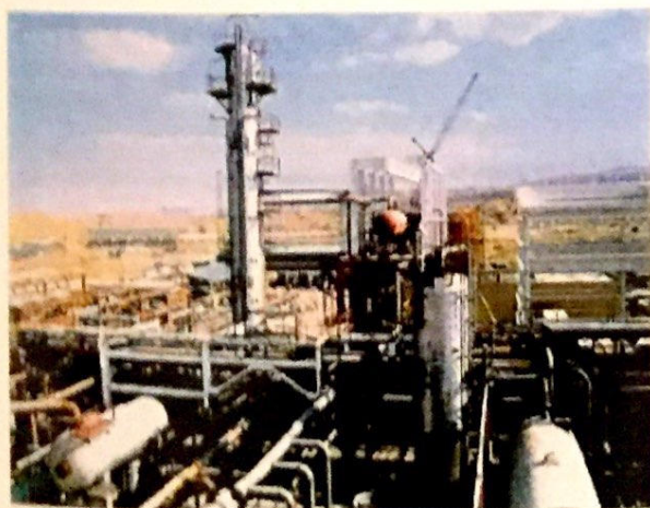
Figure 10: Karaj NLG 1500 Plant (Courtesy of Sazeh Consultants)
