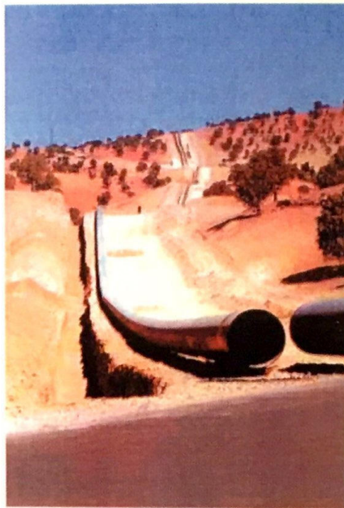
Figure 15 - 56" IGAT 3 Gas Trunkline (Courtesy of Tehran Jonoub)
