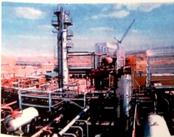
Figure 10 - Karanj NGL 1500 Plant (Courtesy of Sazeh Consultants)
